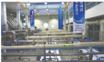
Yeongdeungpo Drinking Water Treatment Plant in Seoul Client ----- Seoul City Capacity ----- 25,000m 3 /day
