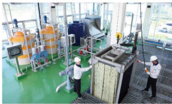
Jeungpyeong Industrial Complex Wastewater Treatment Plant Client ----- Jeungpyeong City Capacity ----- 2,500m 3 /day
