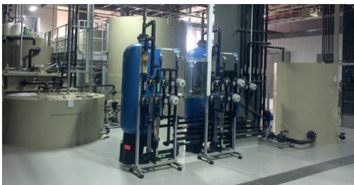
Picture 1. Physical chemical treatment plant
