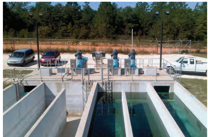
Figure 3: MBR treated water clearwell
